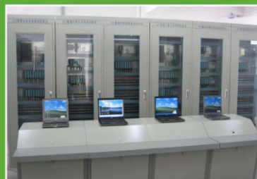
▶ DCS控制系统
